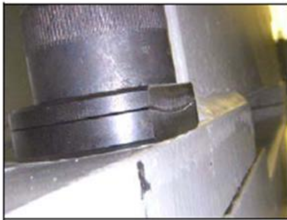
Figure 2: Counterweight Bolt/Washer Inspection
